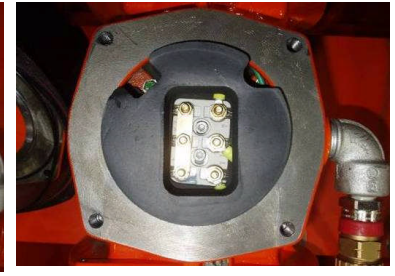
Figure 27 Thick Isolator - Motor Leads Not Showing
