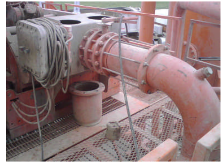
Figure 10 Inlet Pipe & Flange Connected to Header Box
